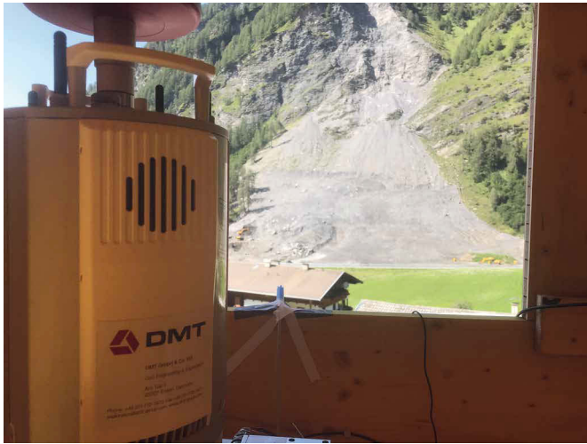
Fig. 3 Setting up the scanner on a measuring point in a shelter in the Vals Valley.
