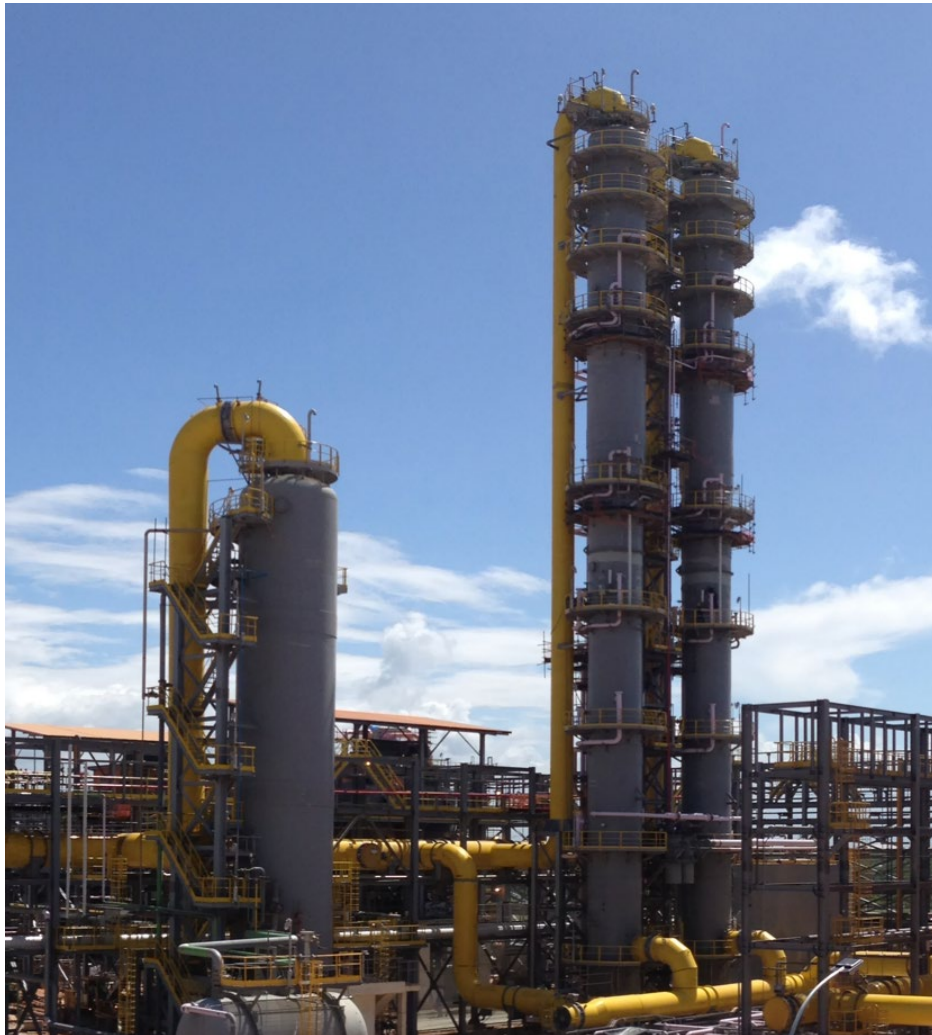
H 2 S/NH 3 -Combi- Scrubber 83,000 Nm 3 /h
