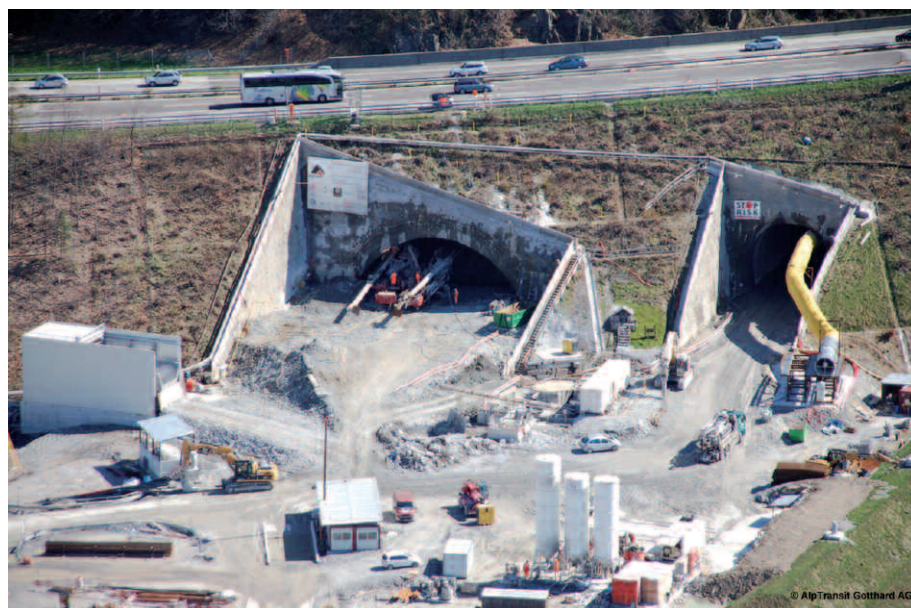
Fig.1: Vigana: View of the Vigana north portal, over which the A2 passes – one of the two main traffic axes through Switzerland.
