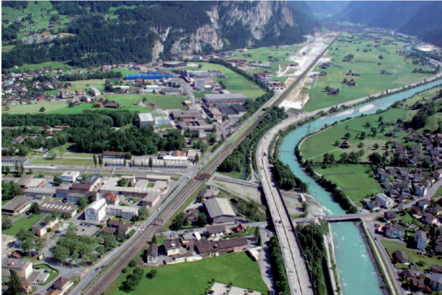
Fig. 1: Overview of the construction site of Altdorf/Rynächt up to the section of Erstfeld.
