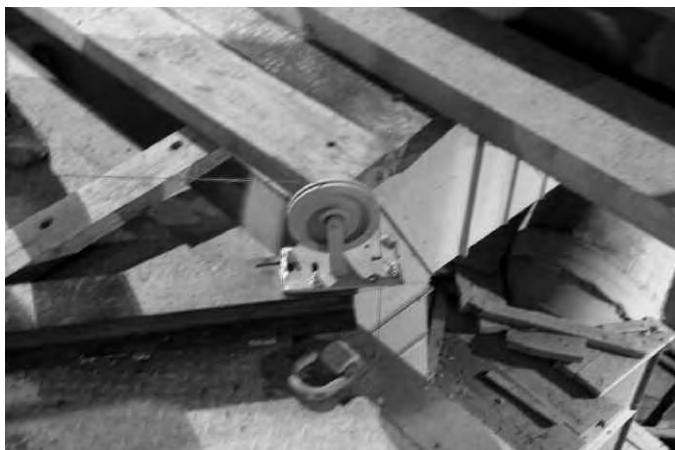
Fig. 6: Deflection pulley with plumb wire.
