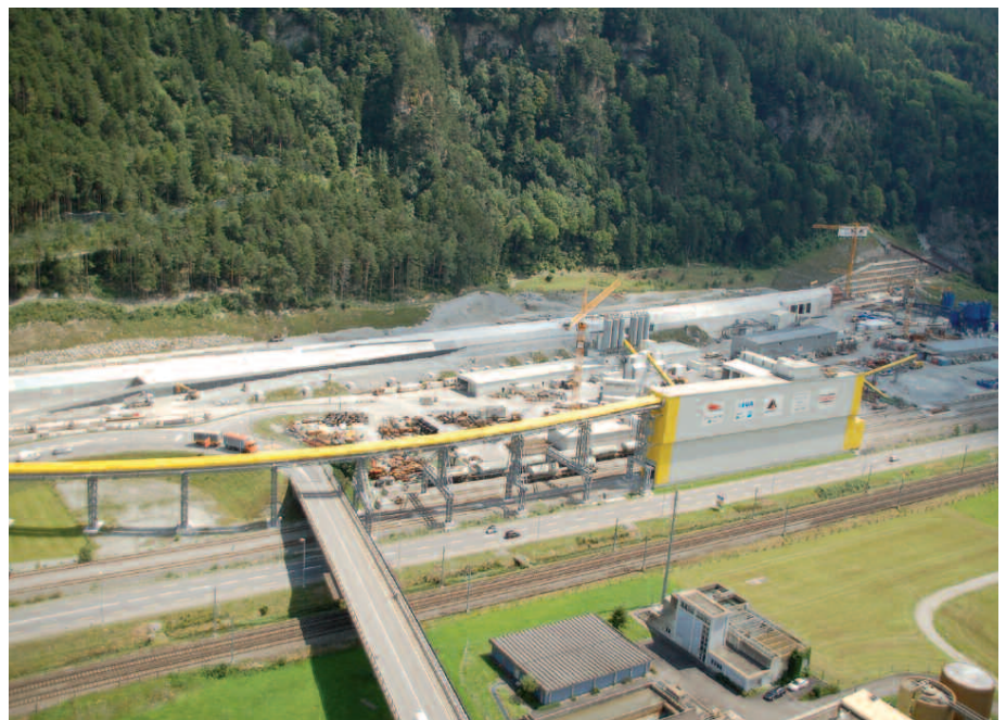
Fig. 1: The portal area in Erstfeld: The drilled pile retaining wall on the right secures the mining slope area immediately in front of the tunnel entrance. To the left of it, the surface tunnel has already been created. Conveyor belts and the installation area surround the construction site (Photo: AlpTransit Gotthard AG, Adrian Wildbolz).
