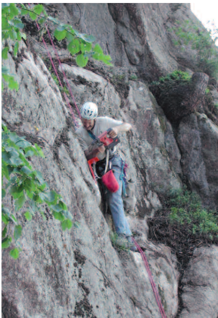
Fig. 3: Attaching the measuring points above the mining tunnel portal (Photo: Basler & Hofmann).
