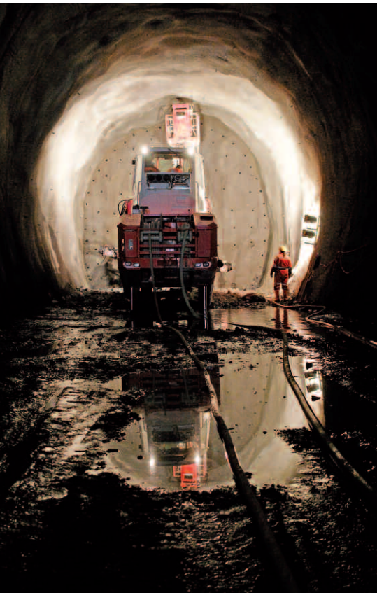
Fig. 5: Drilling holes for blasting by the north portal of the Ceneri Base Tunnel.
