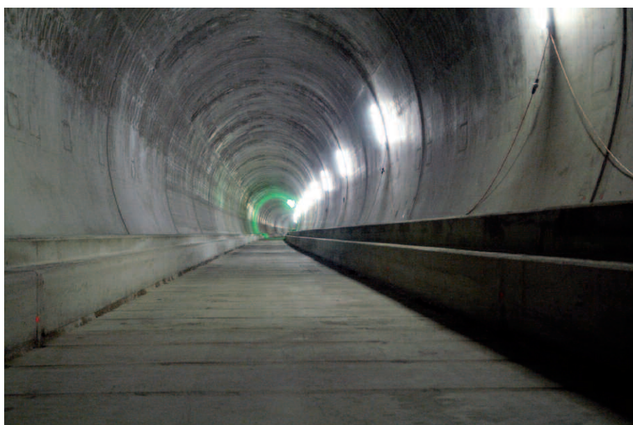
Fig. 4: In May 2010, installation of the railway infrastructure began in the west tunnel in the Bodio section.
