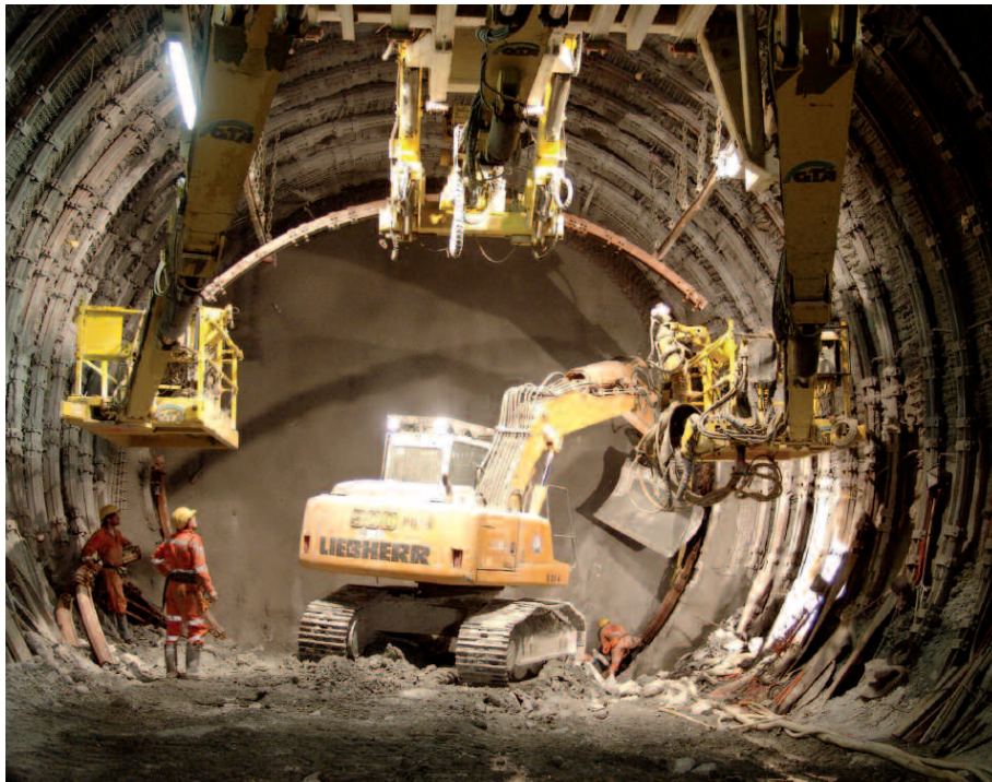
Fig. 2: To stabilise the rock in the Sedrun section, flexible steel rings were installed.
